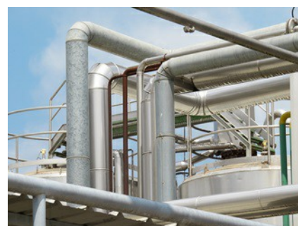
There is not only a lot of pipework on the outside; heating coils and installations also influence the measuring signals inside the reactor.
