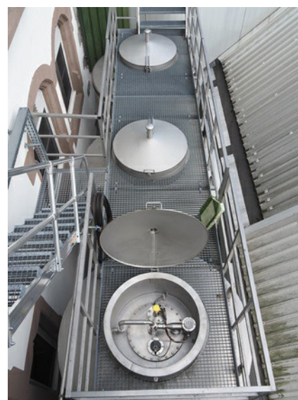
View of a VEGAPULS 63 radar level transmitter on one of the maturation vessels.
