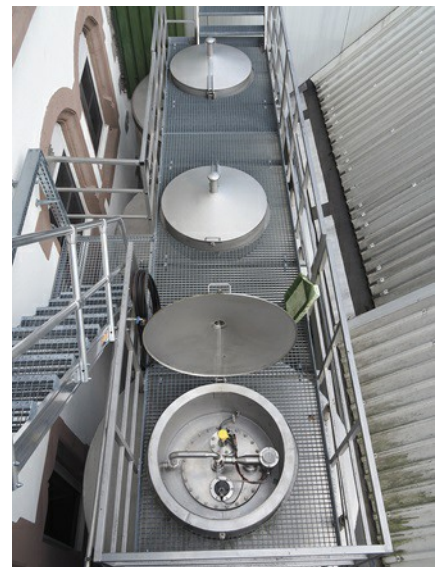
View of a VEGAPULS 63 radar level transmitter on one of the maturation vessels.
