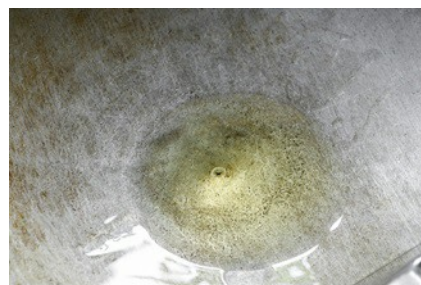
Oil on the tank floor. At low levels, it is very difficult to measure oils or other liquids accurately.
