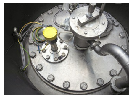
A VEGAPULS 64 radar level transmitter performs contents measurement.
