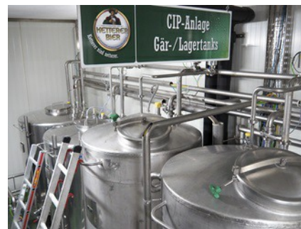
Additional pressure transmitters are used in the CIP tank.
