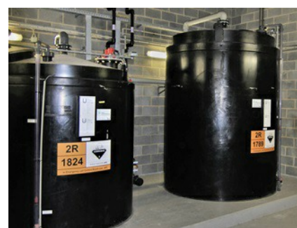
Chemical tanks for storing acids and alkalis.
