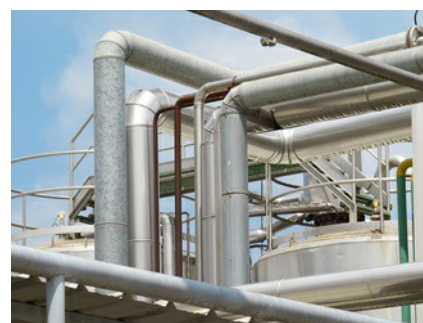
There is not only a lot of pipework on the outside; heating coils and installations also influence the measuring signals inside the reactor.
