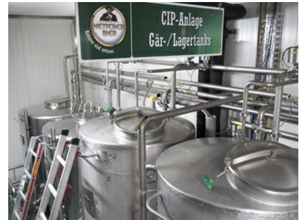
Additional pressure transmitters are used in the CIP tank.
