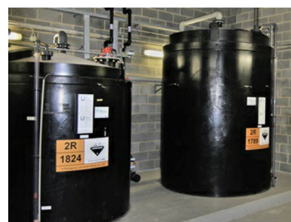
Chemical tanks for storing acids and alkalis.
