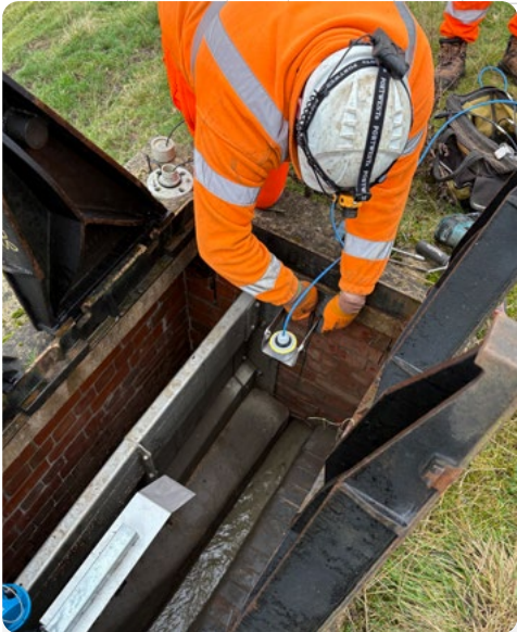
Installation of a VEGAPULS C21 radar level transmitter for spill discharge monitoring, supporting reliable measurement and improved visibility of wastewater network activity.
