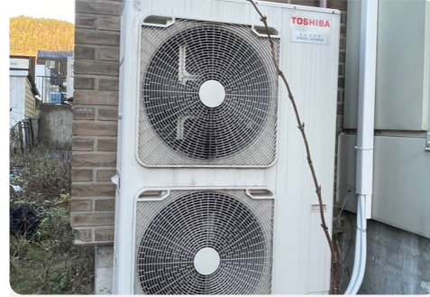
Heat pump at VEGA Norway
