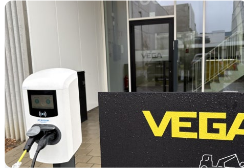
Electric vehicle charging station at VEGA Belgium
