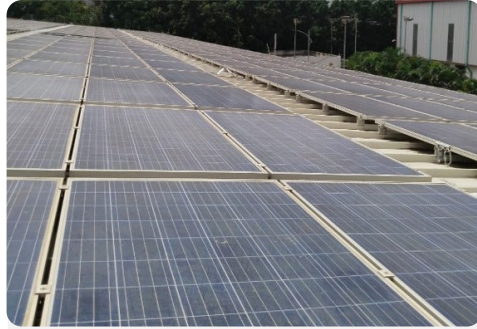
Photovoltaic system at VEGA India
