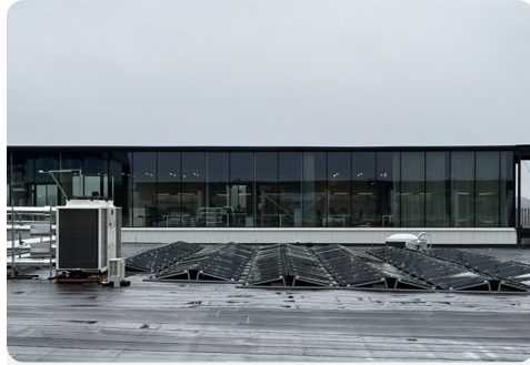
Photovoltaic system at VEGA Belgium
