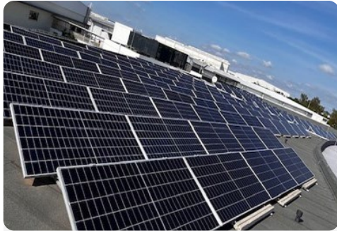
Photovoltaic system at VEGA South Africa
